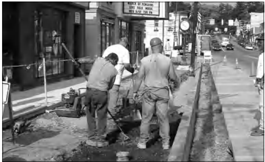
Structural soils can be used under new sidewalks and parking lots, especially those being removed and rebuilt.
